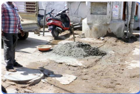
Unrepair Road at Masjid Circle Vemukunta (Before)
