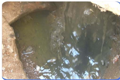
Manhole without cover at Vemukunta
